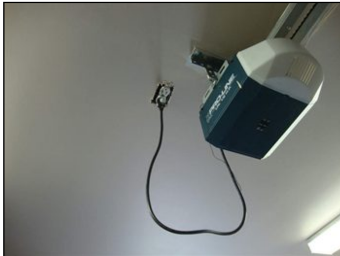
Missing Cover Plate.
