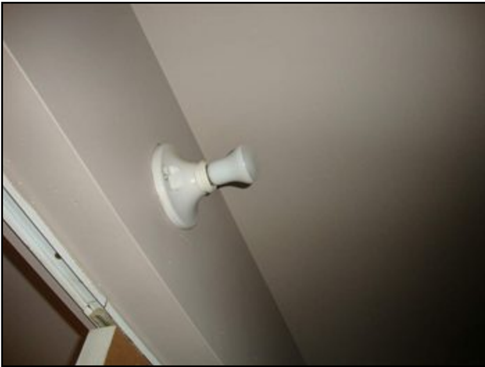
Exposed Bulbs Not Allowed In Closets.
