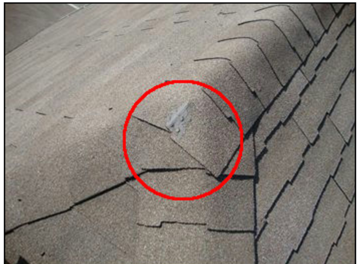
Exposed Nail Heads
