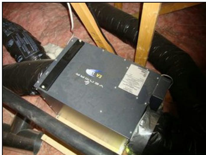
HRV In Attic
