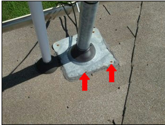
Flashing Installed Wrong.
