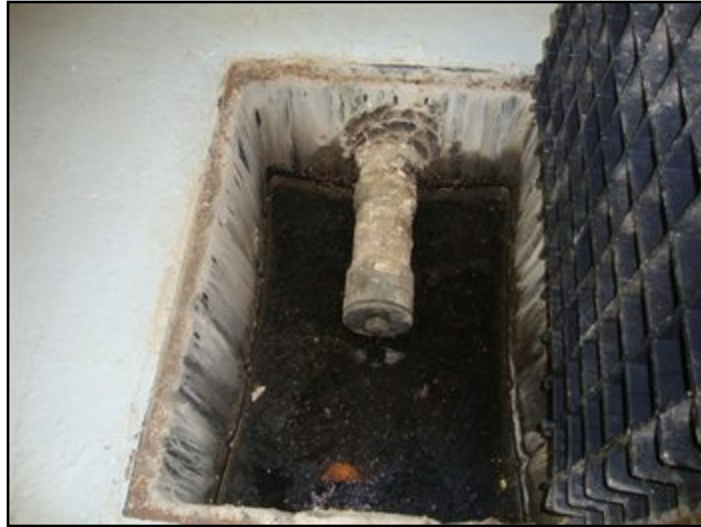
Clean Floor Drain.
