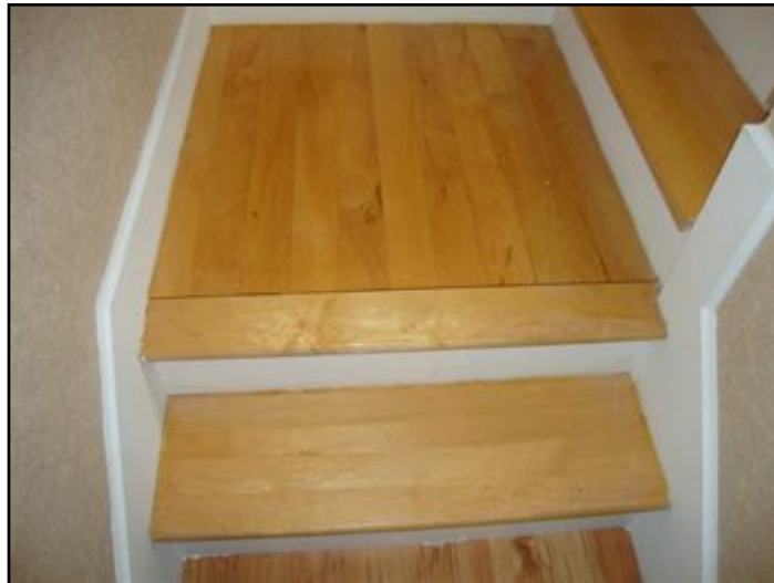
Stair Nosing Has Moved.
