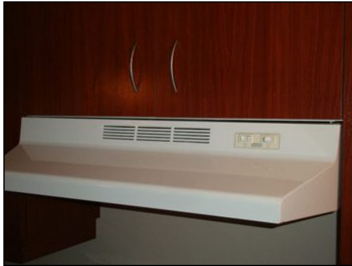
Fan Does Not Vent Outside.
