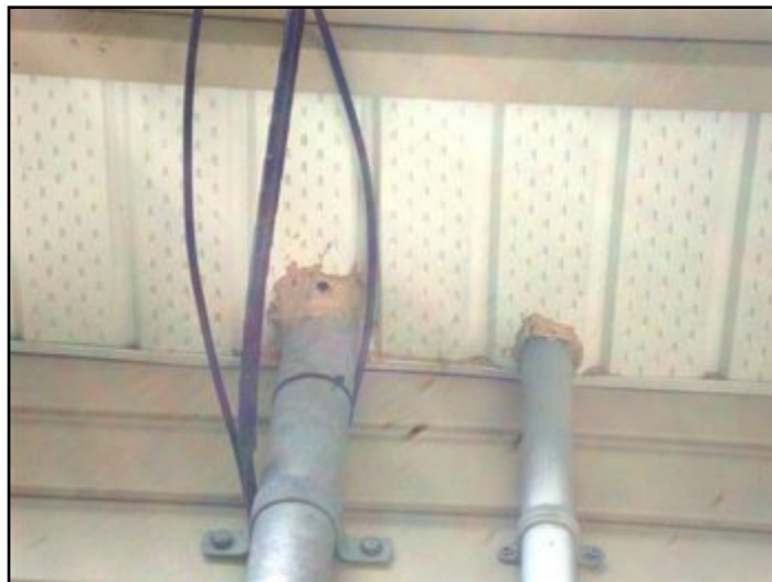
Caulking Repairs Required
