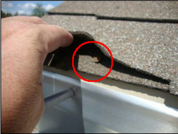
Exposed Nail Head On Edge
