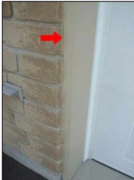
Caulking Repairs Required.
