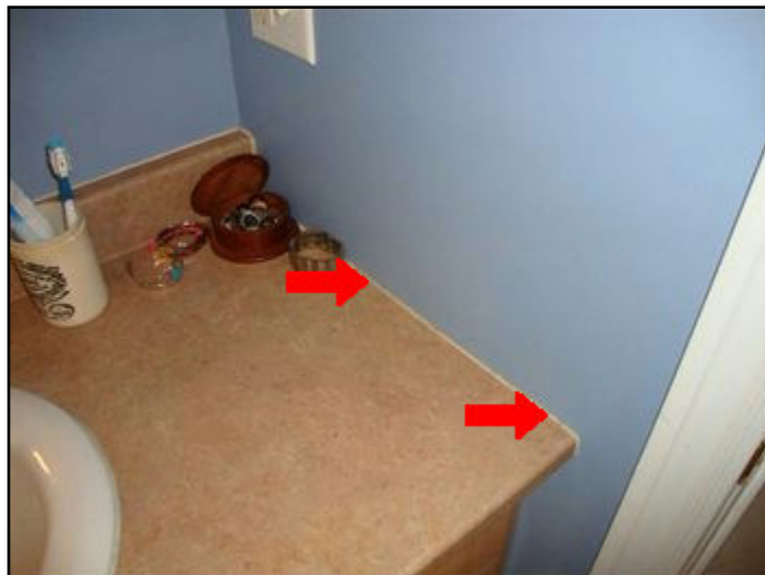
Caulking Repairs Required.
