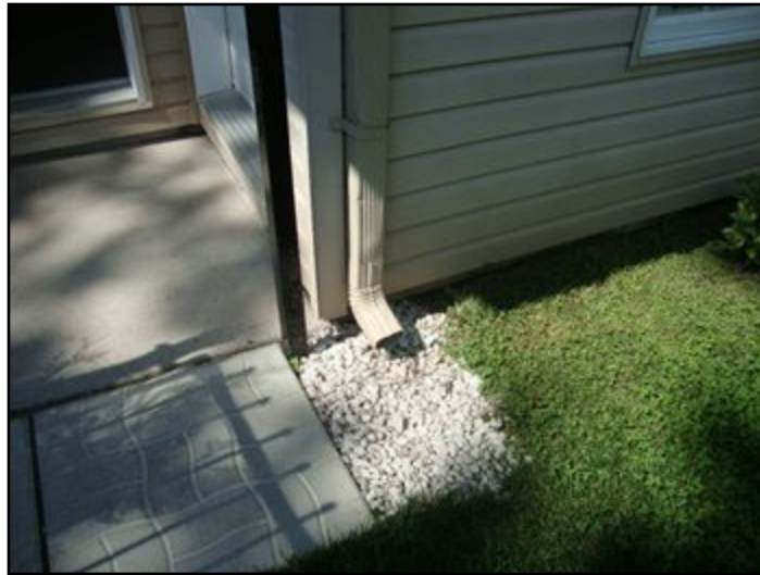
Extend Away From The Building.
