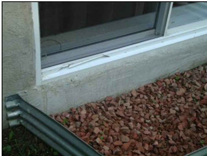
Damaged Window Frame.
