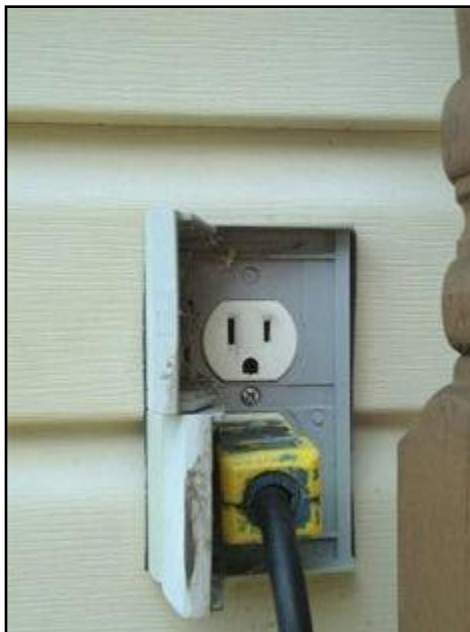
Outdoor Plugs Should Be GFCI Protected.
