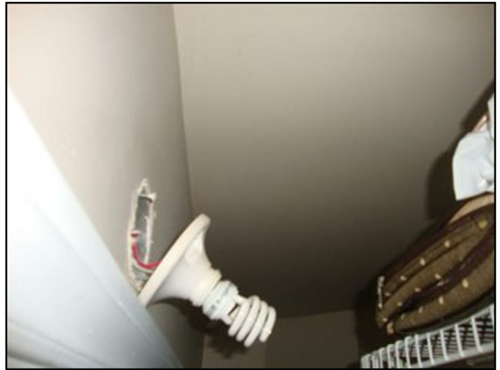
Fixture Not Properly Secured.
