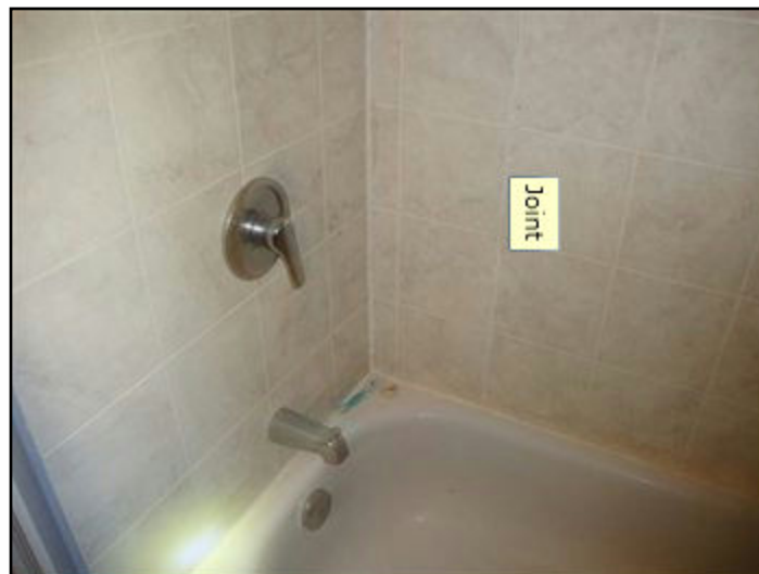
Shower Walls Are Not Tiles.
