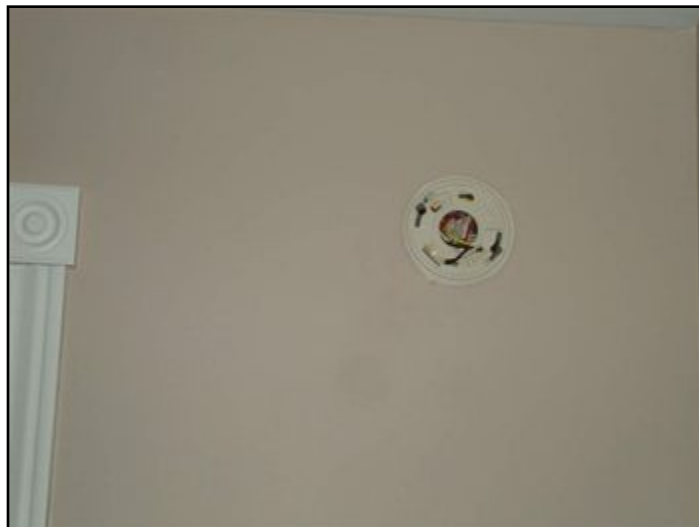
Smoke Detector Missing
